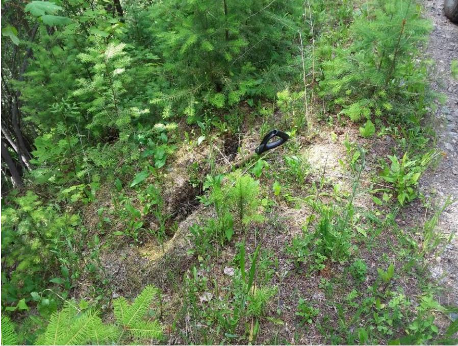
Photo 1 Fillslope Tension Crack at Sal 50.
